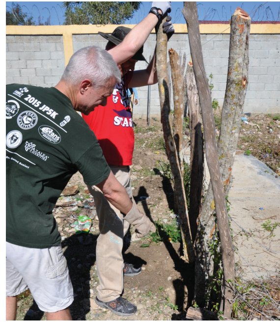
Andy & Fr. Christensen help build property fence line at St. Clare Chapel
